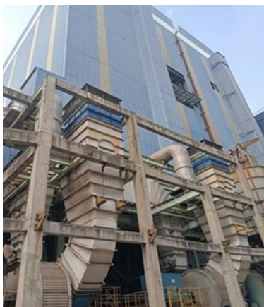
Gambar 1. Boiler CFB MB 26
